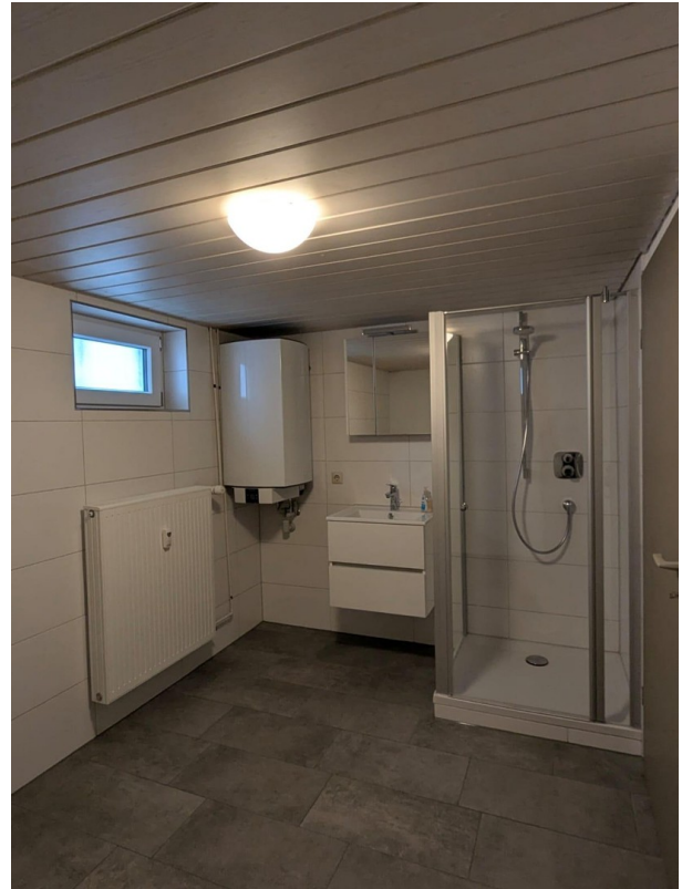
Bad Zeile komplett / Boiler
