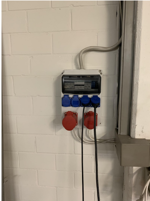
Strom Lager H
