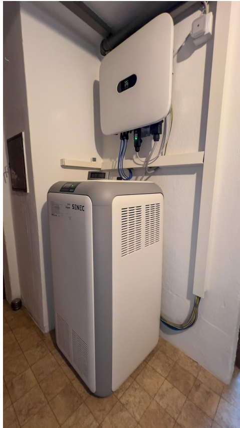
10 kWh LFP Akku Speicher
